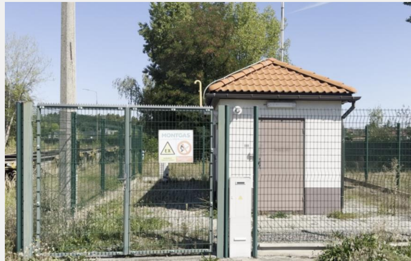
Gas distribution station
